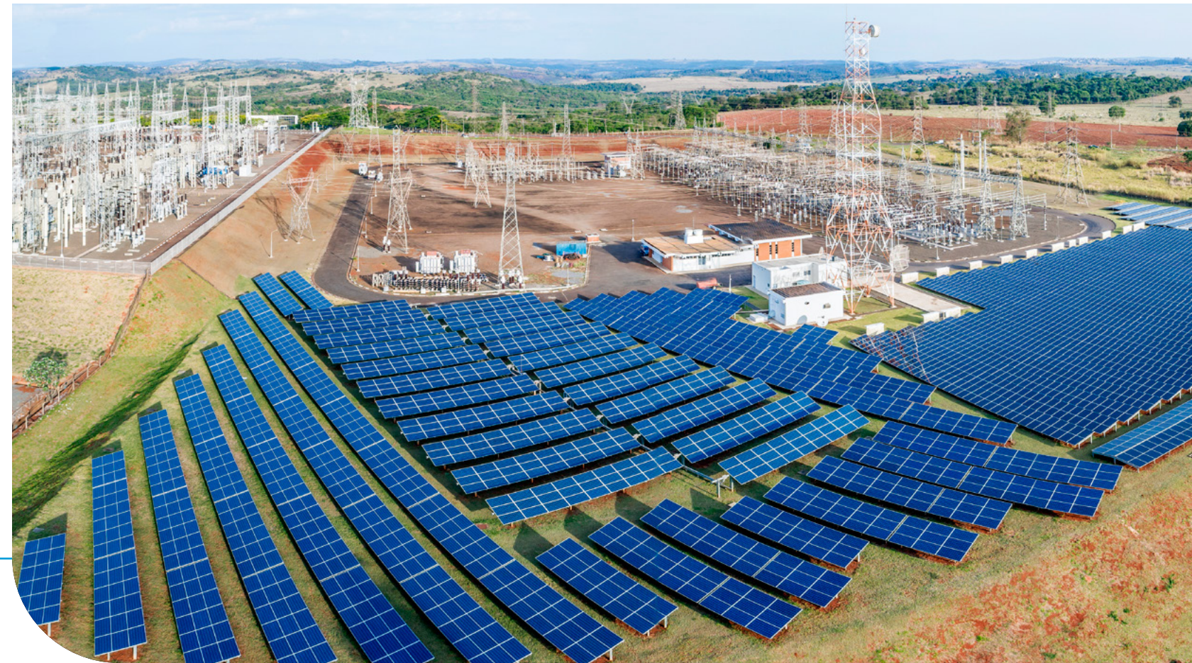
Tanquinho Solar Power Plant, in Campinas (SP).
