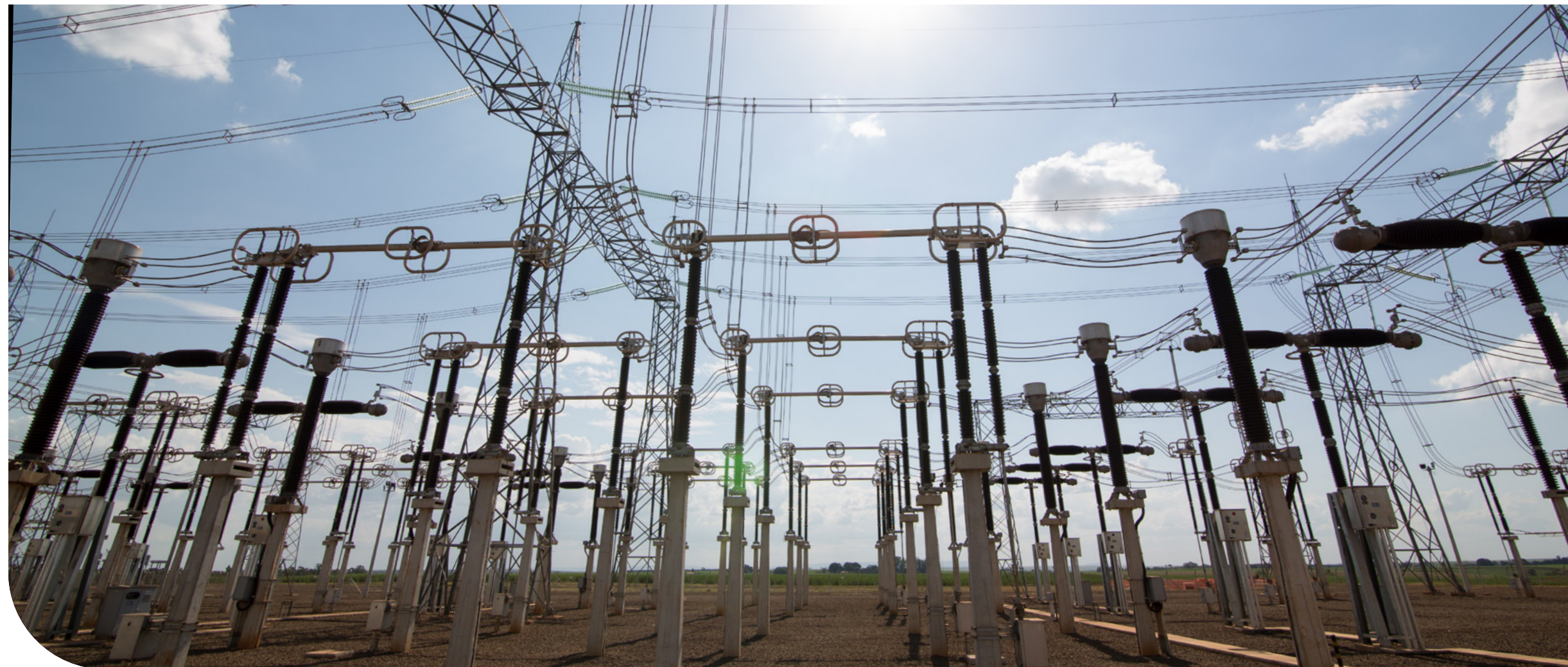
Piracicaba Substation, in São Paulo.
