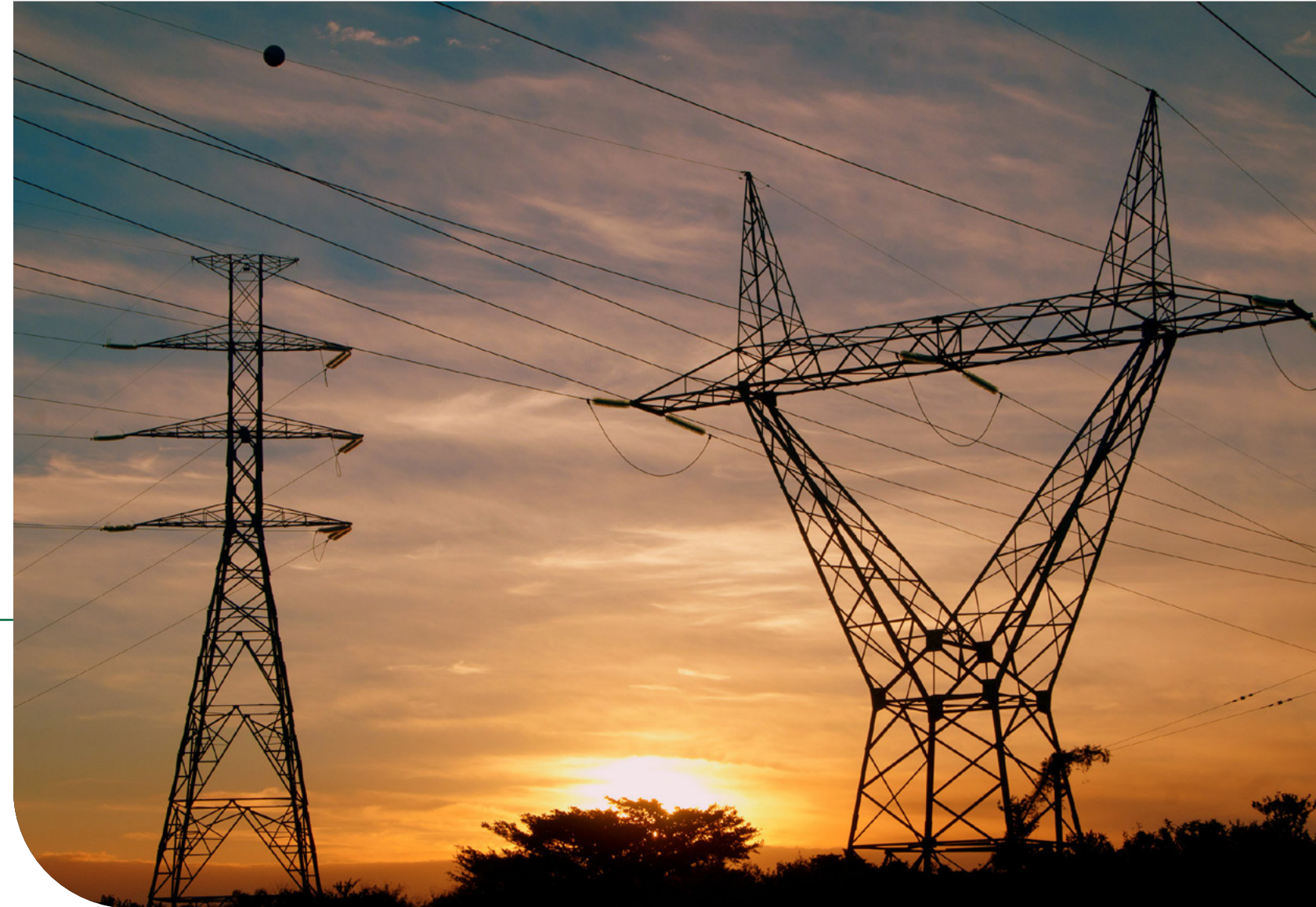
Transmission line in Rio Grande (RS).
