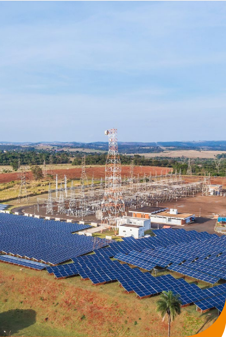
Tanquinho Solar Power Plant - Campinas - SP
