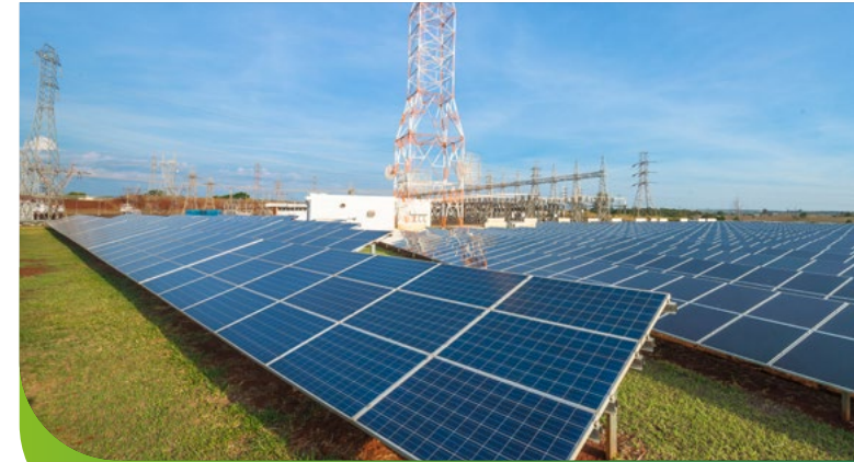
Tanquinho Photovoltaic Plant in Campinas - SP
