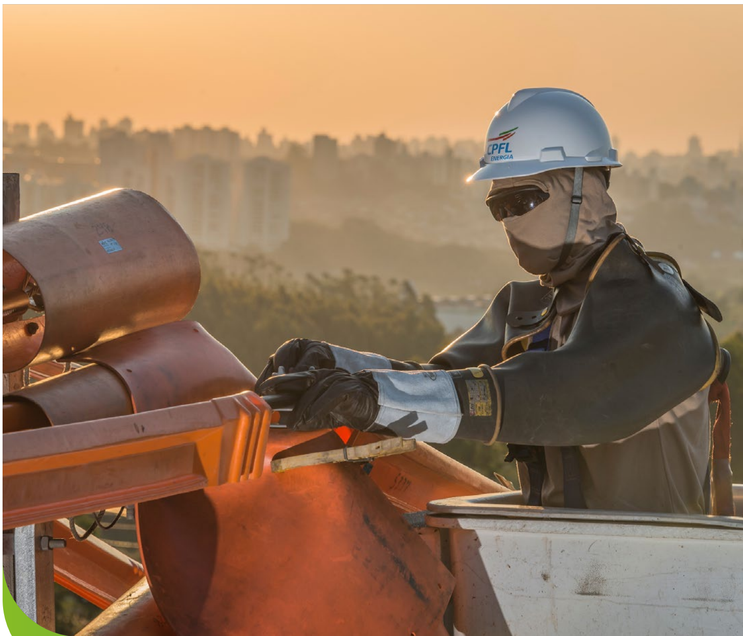
Employee at CPFL operation
